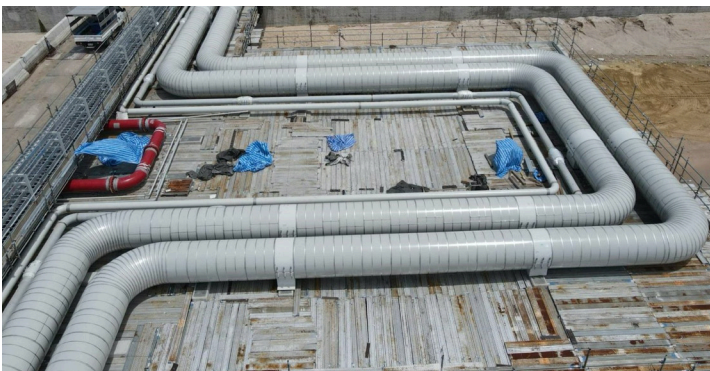
Figure 3. LNG terminal in Thailand shows a fully insulated contraction loop enjoying a reduced dressed-out final dimension in comparison to standard duty insulation materials.
