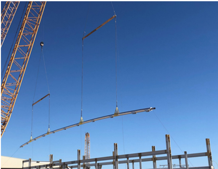
Figure 2. Fully insulated with Cryogel Z and a vapour barrier, these nearly 300-ft-long sections were assembled at ground level and hoisted into racks. The flexible design of Cryogel Z was the only solution trusted to enable the offsite fabrication for this project.
