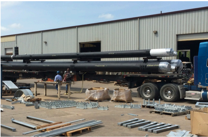
Figure 1. Cryogel Z pipe spools fully insulated and vapour sealed. After a 1000 mile trip, these pipes showed zero failures of the insulation system. In comparison, the rigid system showed multiple areas of condensation, icing, and loss of vapour barrier integrity upon testing.
